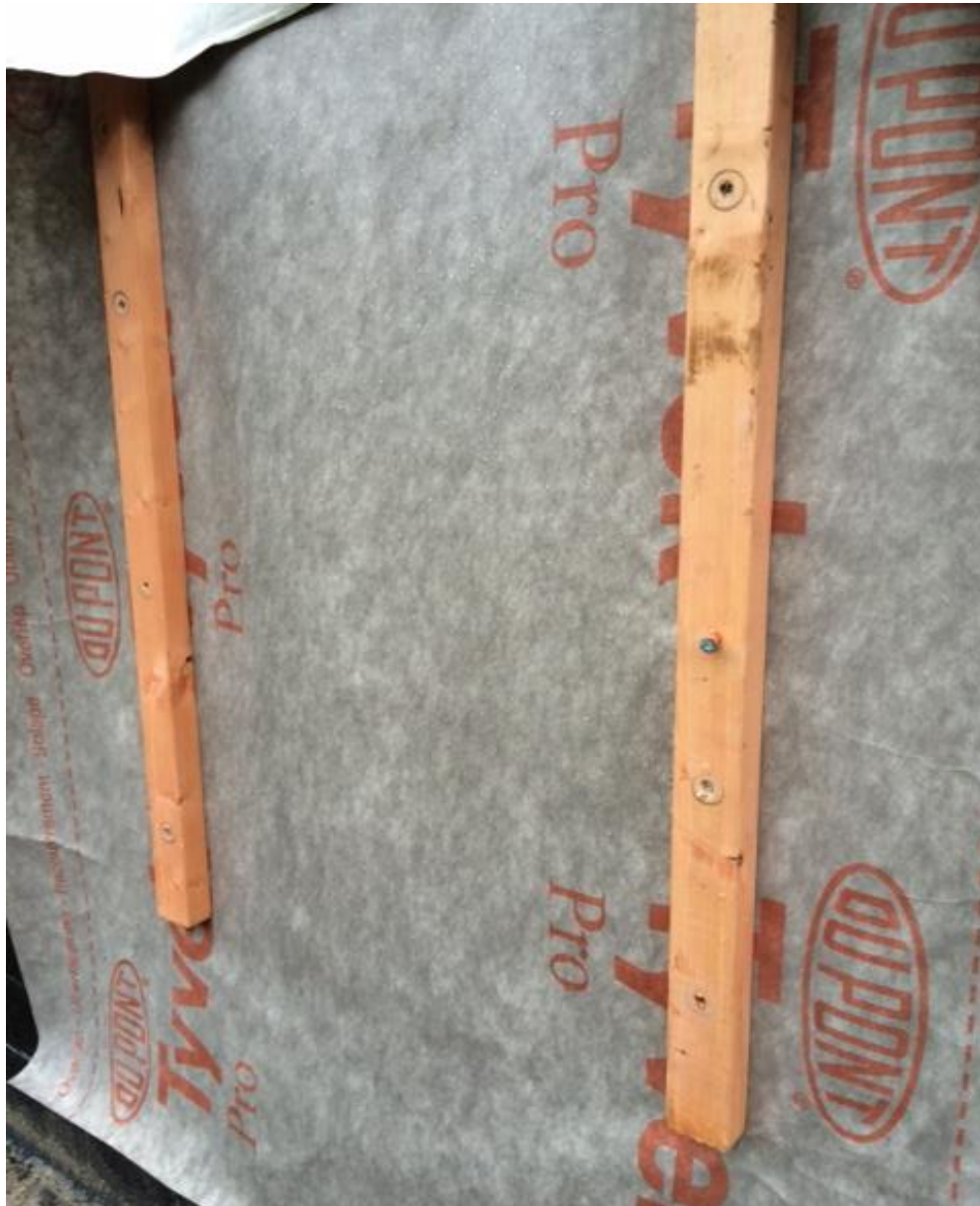
Photo 1/3: detail of perforations trough wall
